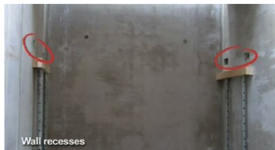
M4: Place the support for the landing, and adjust it to the right height.
