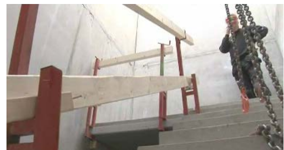
M24: The landing and the stair are finish. Ready for the next floor.
